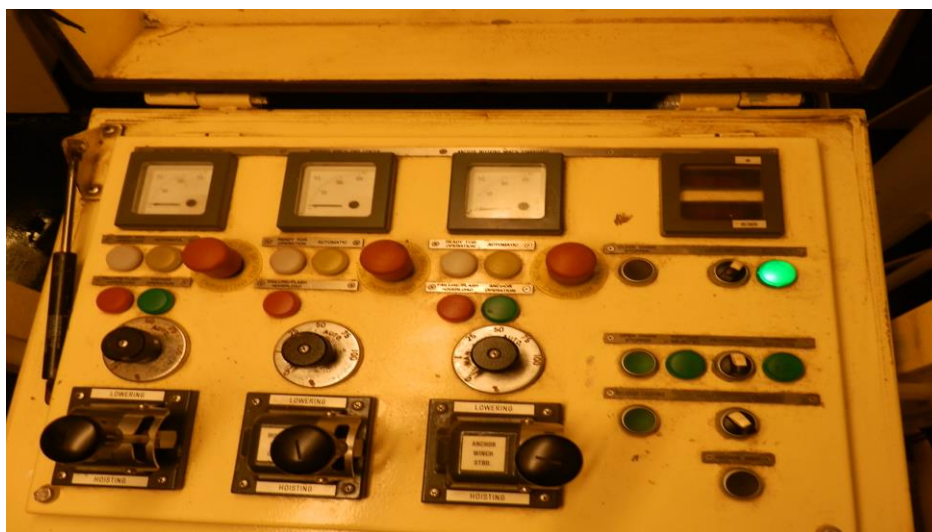
Figure 16. Control panel fitted on control post.
