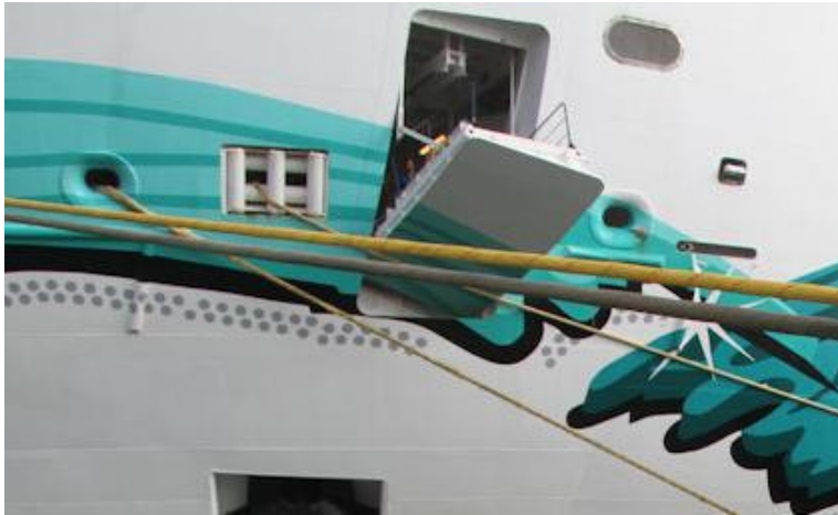
Figure 6. The damaged mooring platform following the marine casualty
